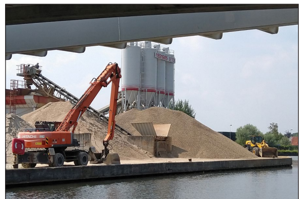
Betoncentrale Mermans in Arendonk
